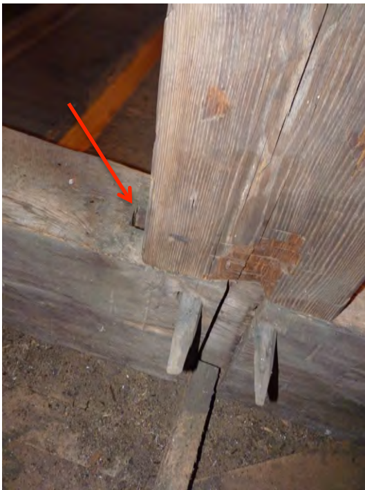
Fig. 22. King post mortised with interlocking tenon into bottom chord of truss. Notice pegs but missing wedge at left and sliding ceiling joist mortise joint.
