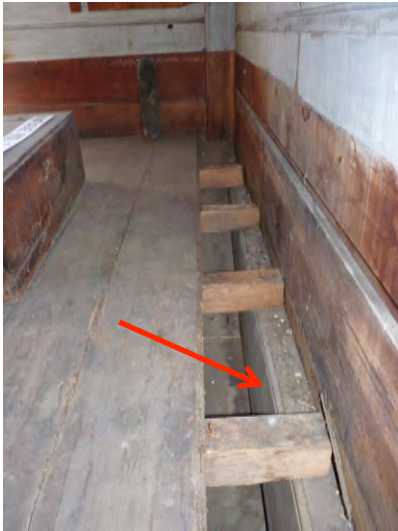
Fig. 4. Southeast corner upper meeting hall with stage floor removed. Note girt (red arrow) completely enclosed with beaded wood
