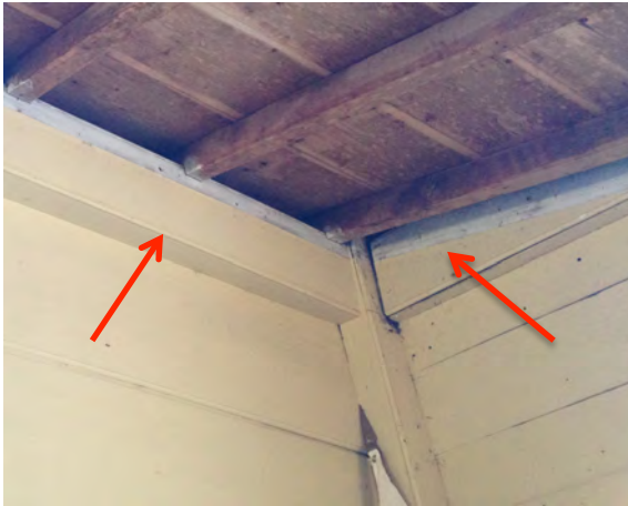
Fig. 5. Southeast corner lower meeting hall looking at gallery floor. Fully enclosed girts with beaded wood trim (red arrow) only occur at the Southeast and Southwest corners. Beaded wood trim extends up and beyond gallery floor joist. See Figure 4.
