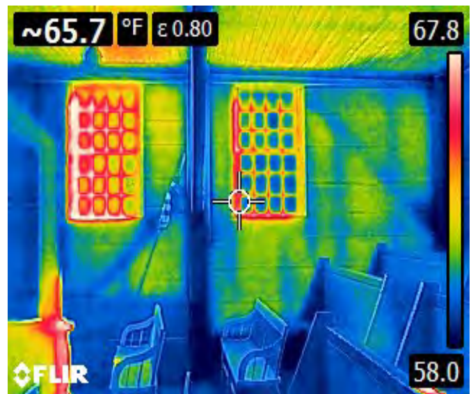
Fig. 21. Interior thermal image of Southerly wall to the right of the stair porch. Locations of wood posts, diagonal braces, wall studs, ceiling joists and ceiling bracing can be clearly seen.
