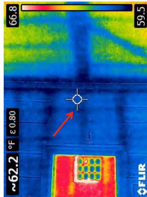
Fig. 5: Upper meeting room entrance door and ceiling above looking into the stair porch. Centered at top is the bottom chord of the timber roof truss above the beadboard ceiling, a diagonal wood brace parallel to the ceiling plane, wood ceiling joists, the south timber roof sill (heavy blue horizontal near top), and vertical wood wall studs. The original door header (red arrow) confirms that the door was higher in order to access the high point of the South gallery floor which was present in 1818.
