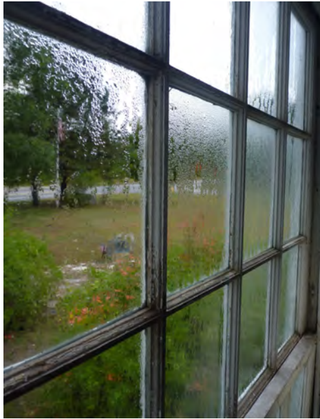
Fig. 13. Condensation forming on interior of 12/12 window causing failure of paint on muntins.
