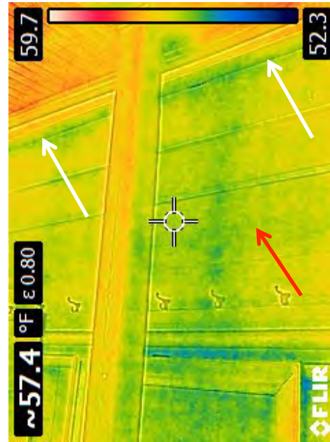
Fig. 7: Upper meeting hall North wall at pulpit window. Parallel to the wall plane and directly above the post in front of the pulpit window is the bottom chord of the timber roof truss. Shown is the North rafter plate (white arrow) and the timber post below that supports the truss above and rests on the pulpit window header. Of interest is the horizontal wood member (red arrow) that is located near the midpoint of the wood wall paneling. Its location near the midpoint indicates it was not installed to support the edge of the paneling. It may be there to brace both sides of the post. Located above the pulpit window, it may have been used to support the sounding board and possibly indicate the sounding boards location. Further investigation is necessary.
